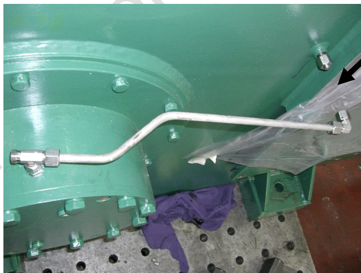
Figure 1: Disconnected hydraulic pipe
